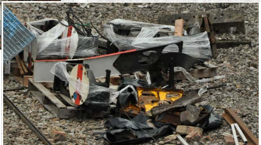
Below—A pile of debris including parts of the old semaphore signals.
